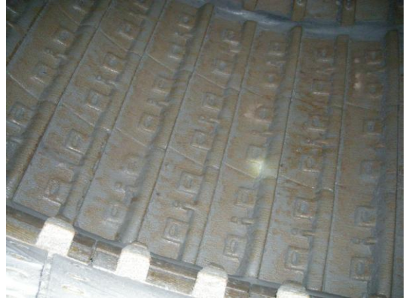
图二 提升条部位严重磨损的筒体衬板 Fig.2 Cylinder liners with serious abrasion in the lifting
